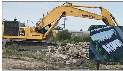
3600 W. 127th Street Construction is underway to develop a new 40,000sqft logistics facility on 8 acres of property that sat dormant for years.
