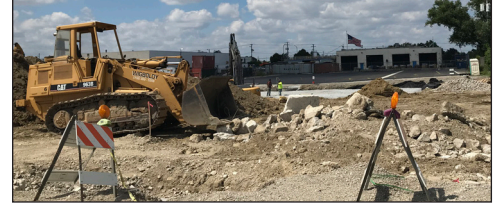
3845 W. 128th Place TarpHaus invested $$ millions to develop a new 5 acre parking lot with the property’s first water retention to eliminate flooding.
